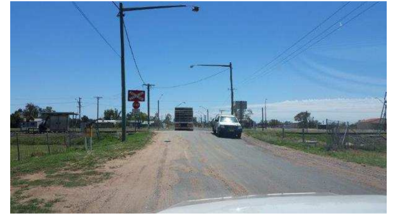
Rail crossing (repair road/reduce grade/seal side-road access / future signalised crossing for improved safety?)
