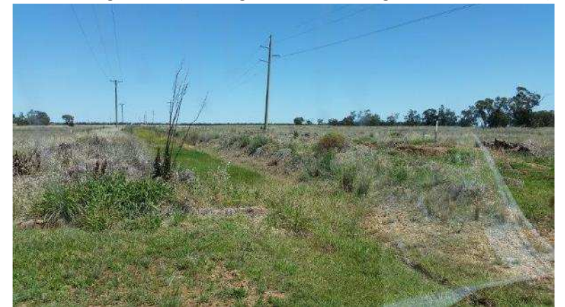
Drain west of Belerenga St (may need releveling to promote drainage)
