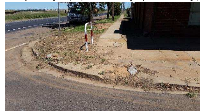
Kerb/gutter Clyde St/Mitchell Hwy needs replacement/extended blisters/new wider footpaths, signage relocation and landscape
